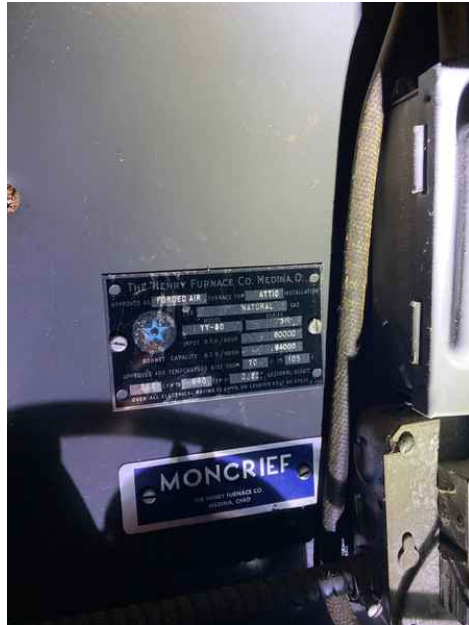
2nd Floor Furnace Data Plate
