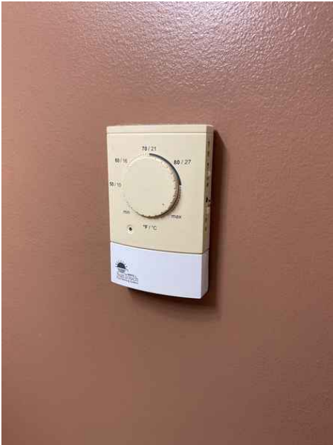
Thermostat/Bathroom in floor heating
