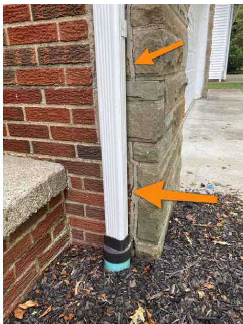
Stone Mortar Cracking
