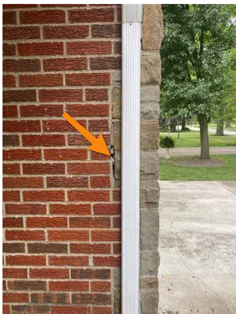
Stone Mortar Cracking
