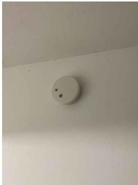
2nd Floor operational
