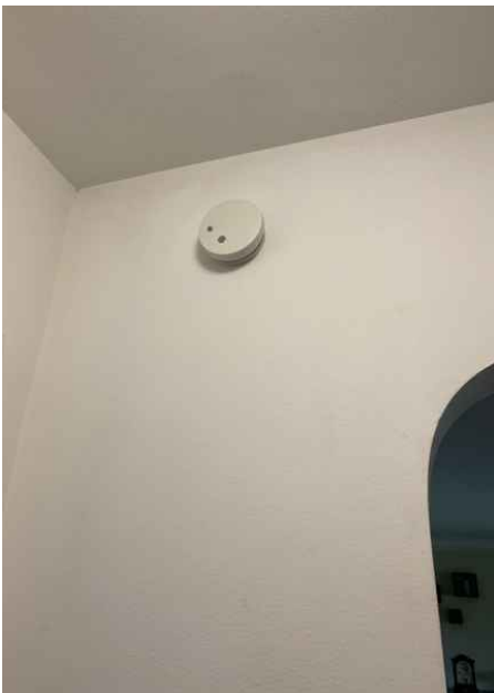
1st Floor Hallway Operational
