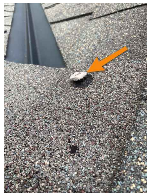
Compromised Sealant front
