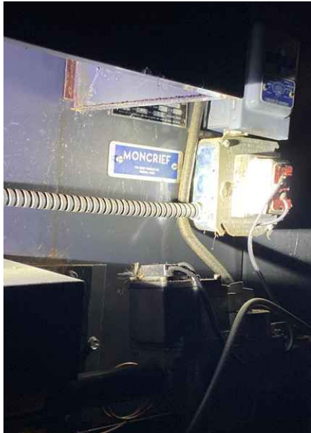
2nd Floor Furnace
