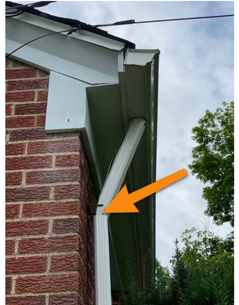
Restricted Downspout Right Rear
