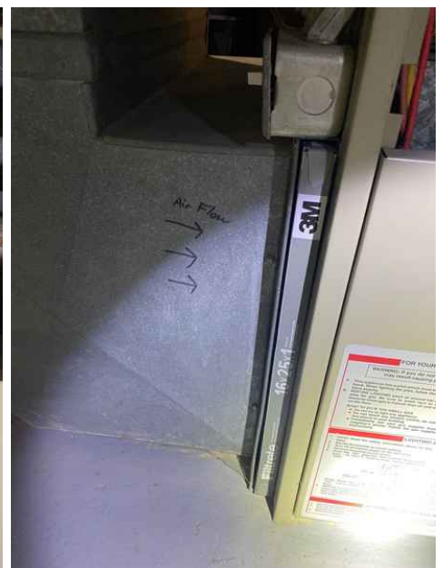
Basement Air Handler Filter
