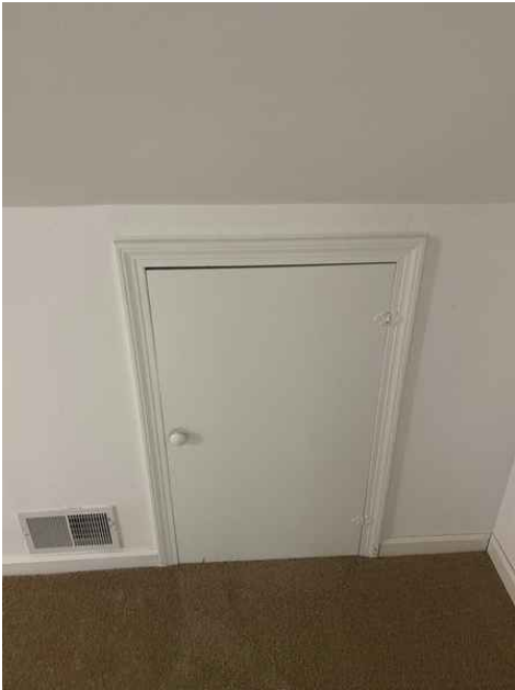
2nd Floor front attic access won't open
