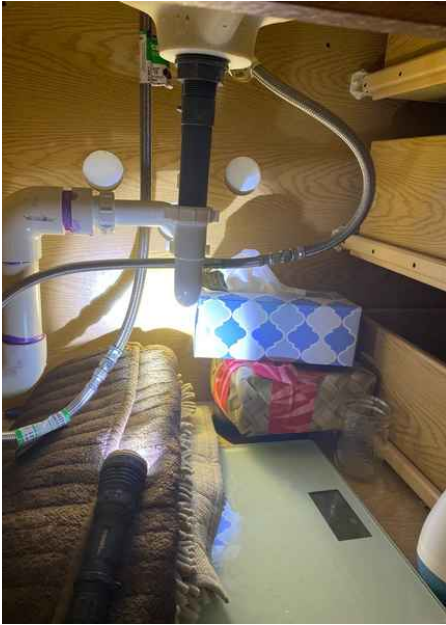
Sink Drain Connections
