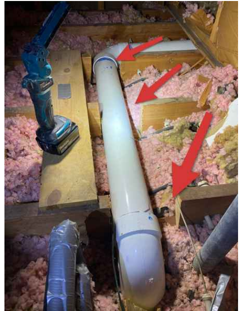
Compromised Ceiling Joists/ Attic Rear
