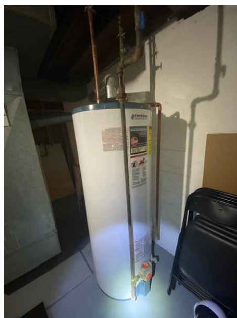
Hot Water Tank
