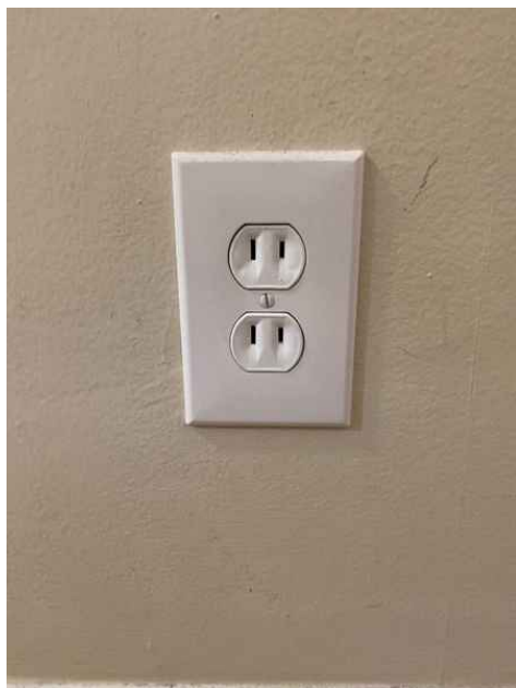
Ungrounded 2 prong outlets throughout house
