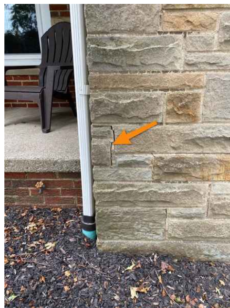
Stone Mortar Cracking
