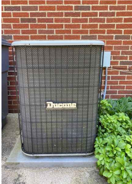
Exterior AC Condenser/Right Side
